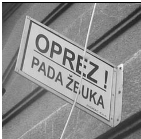
Caution! Plaster falling
