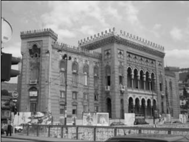
The walls of the National Library (formerly the Town Hall) in Sarajevo, all that is left standing of the library after it was shelled and burned during the war.
